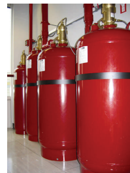
FM-200 fire suppression system instantly eliminates the threat of fire or smoke damage.
