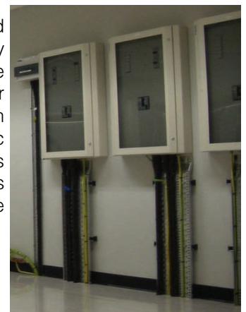
Diverse power feeds ensure multiple resilient supplies can be fed to cabinets.
